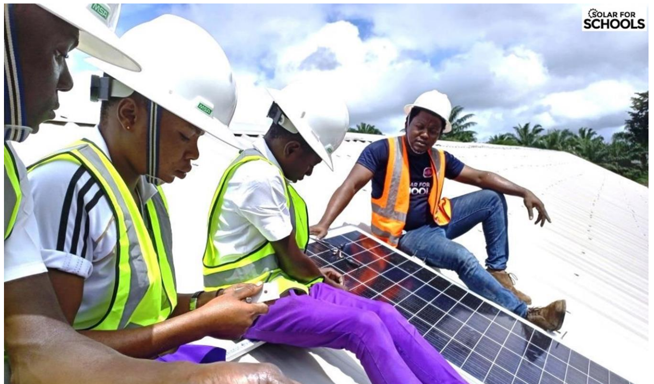
Students installing a solar panel on a roof top under the supervision of the project engineer
