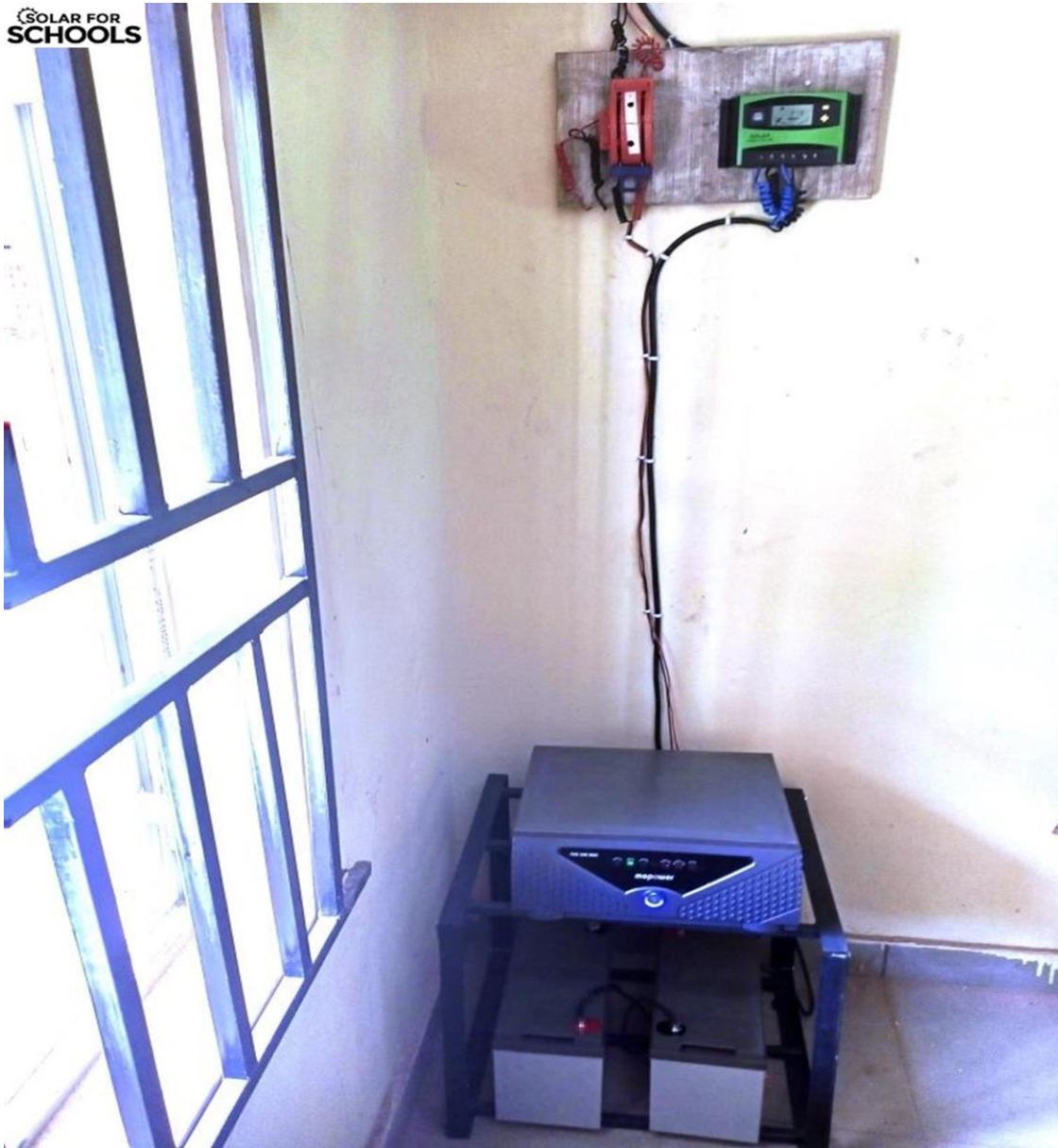
Picture showing the Inverter, charge controller and batteries of the system
