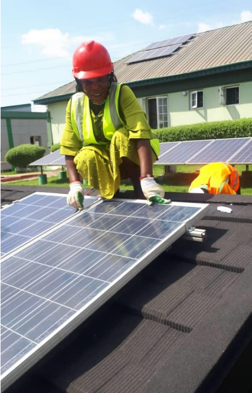
A beneficiary poses for the camera right after installing a panel on the roof
